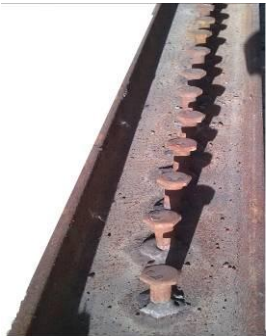
Plate1: The steel channel with its attached headed studs for beam TB –U45
