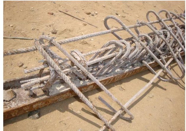
Plate 7: The steel channel and the attached headed studs of the damaged beam TB-U90 after removal of reinforced concrete , showing deformations of the studs .
